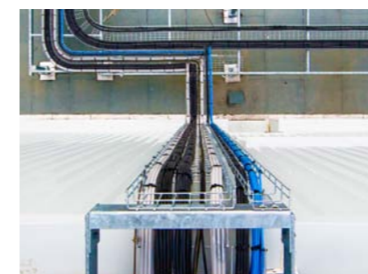
Kabeltrasse | Cable routing
