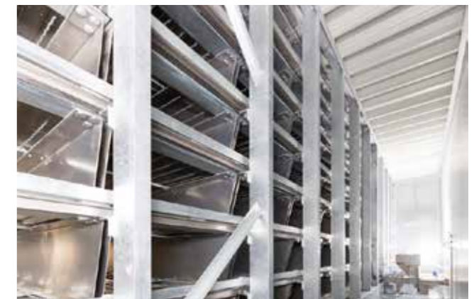
Schockfrostanlage, Kompetenzzentrum AAT, Bereich AAT-FREEZING Blast freezing system, AAT competence center, AAT-FREEZING division
