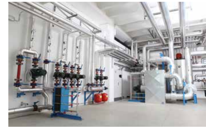
GWH-Installationen, Kompetenzzentrum BT-Anlagenbau, Abteilung HSE-team GWH-Installations, BT-Anlagenbau competence center, HSE-team department
